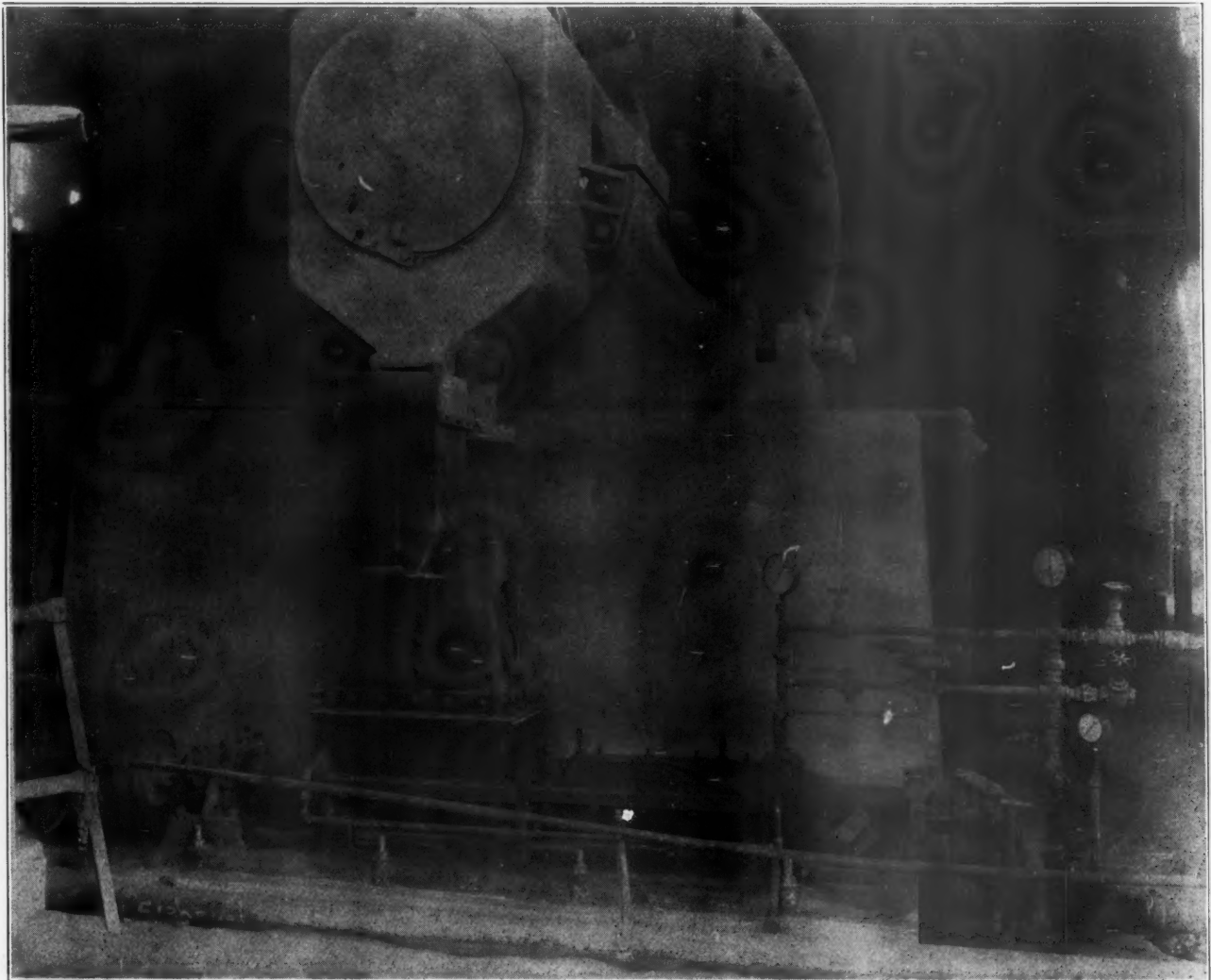
Side View of Pump Showing Air Line From Reservoir
